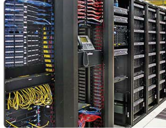
UPS (Uninterruptible Power Supply Systems)
